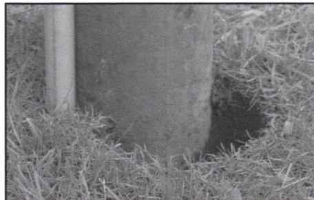
Faulty annular seal.
