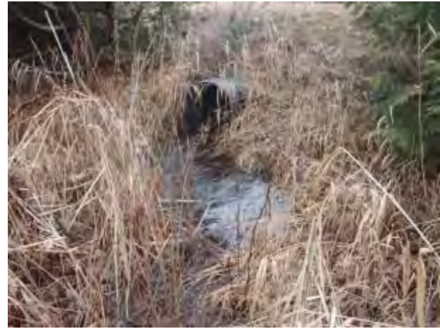
Photo 20: Culvert crossing the municipal access road into the landfill site, that drains the wetland to the north along a ditch to the south.
