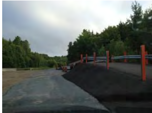
Photo 23: New paved ramp and weigh station installed at the entrance to the landfill.
