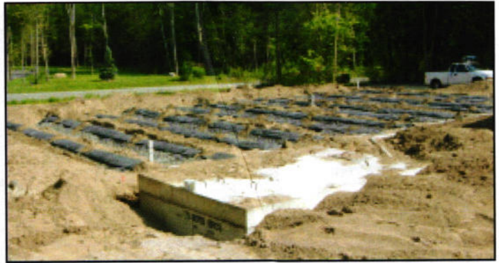
Septic tank and leaching bed.
